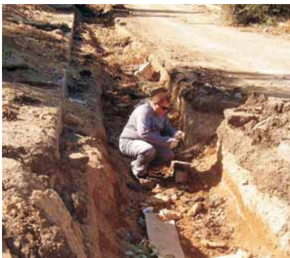
Excavations made to remove power cables for scrap
