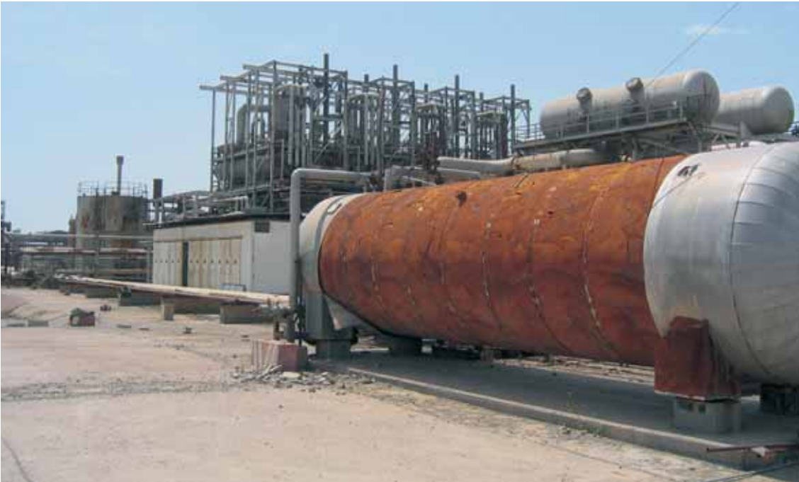
Sulphur purification plant at Al Mishraq
