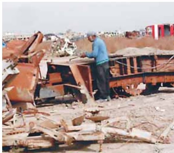
The cutting up and removal of scrap at Quireej was largely uncontrolled
