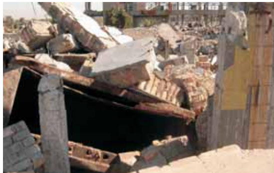
Site after demolition showing destroyed chemical wash tank
