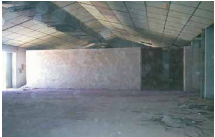
The mercury storage warehouses is now largely empty with a thick layer of chemical dust spread on all surfaces
