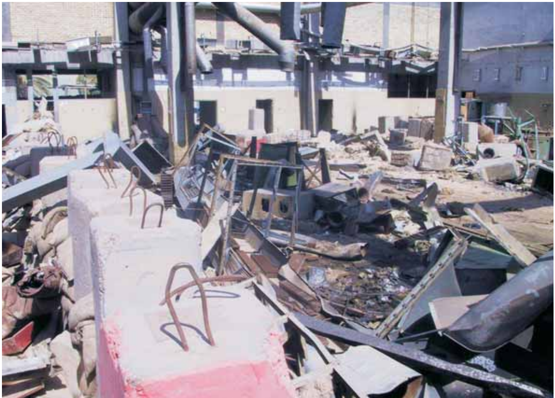
Conflict damage to the Al Qadissiya plating works
