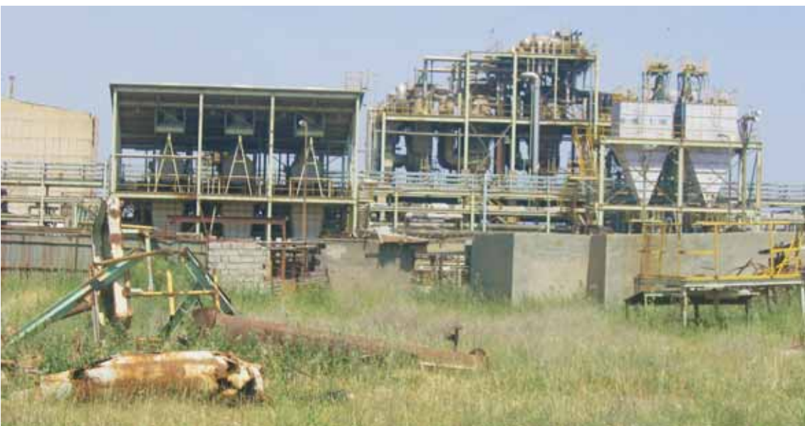
The sulphuric acid plant is in poor condition
