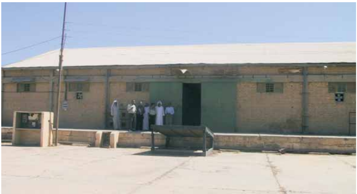
The warehouses storing cyanide compounds are intact but currently too hazardous to enter without protection
