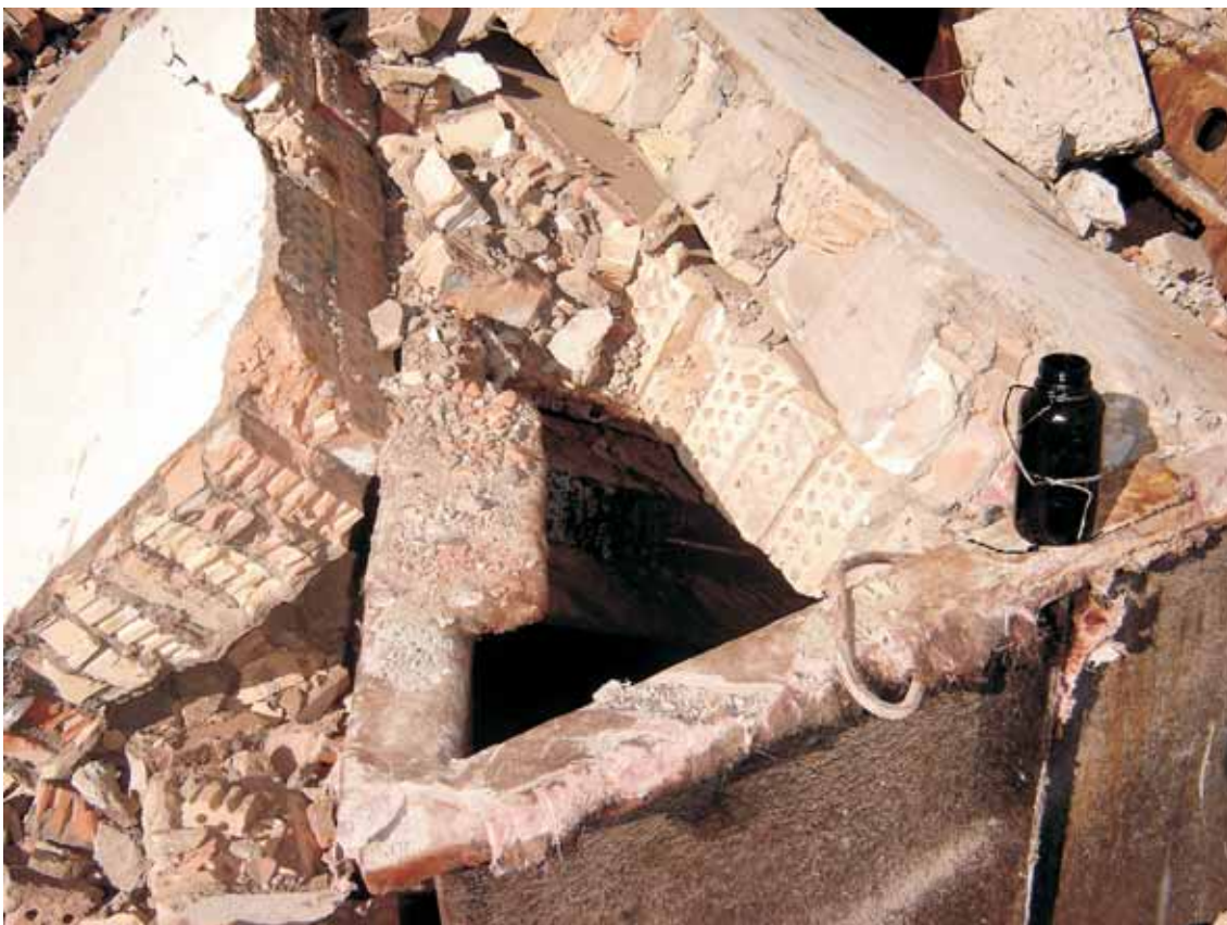
The uncontrolled demolition has resulted in the mixing of inert waste such as bricks with hazardous waste such as the contents of damaged reaction vessels
